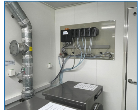
Automated dosing system for laundry
